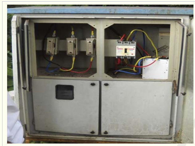
Street Light Control System
