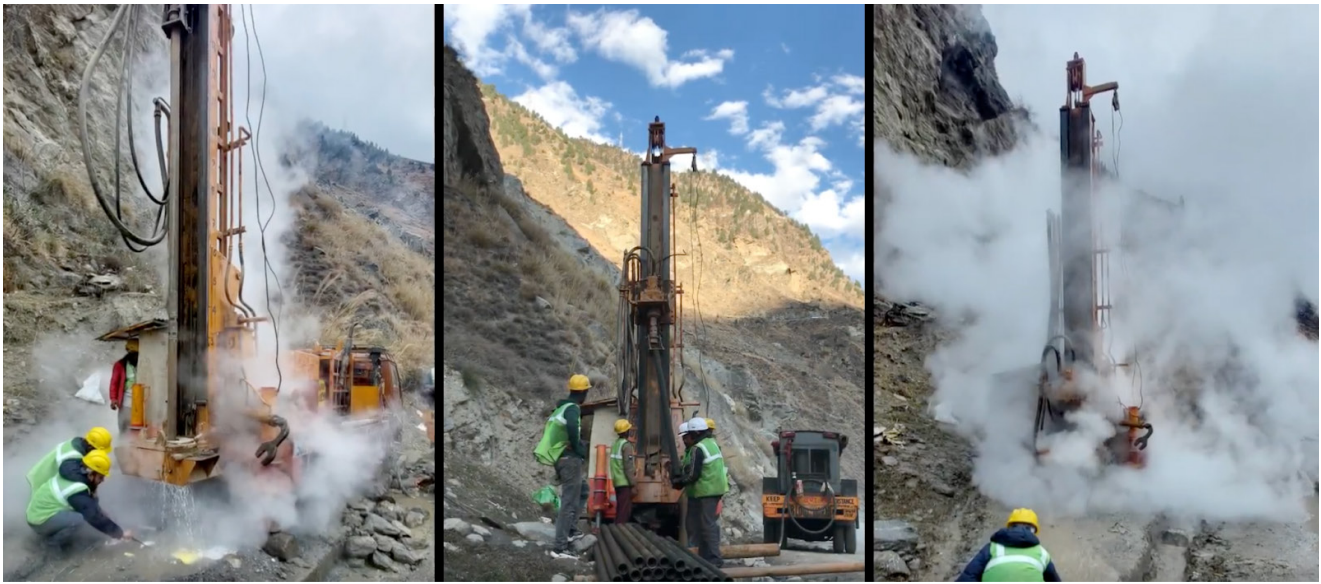
Figure ES.9: The Tapri Geothermal Cold Storage Project, an InnerSpace GeoFund portfolio project. Source: Geotropy.
