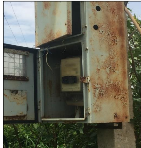
Figure 8: Meter not connected
