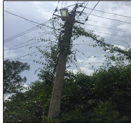
Figure 12: Overhead lines covered with bushes
