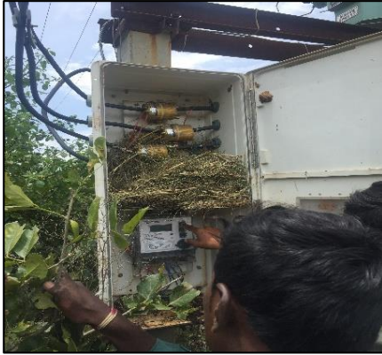
Figure 14: Poor condition of DT meter
