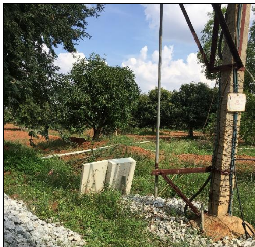
Figure 24: Illegal connection of IP set to NJY feeder
