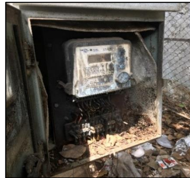
Figure 17: Poor condition of meter box and faulty meter
