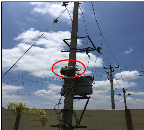
Figure 9: DT meter placed high
