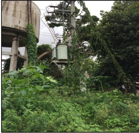
Figure 11: Transformer covered with trees and creepers
