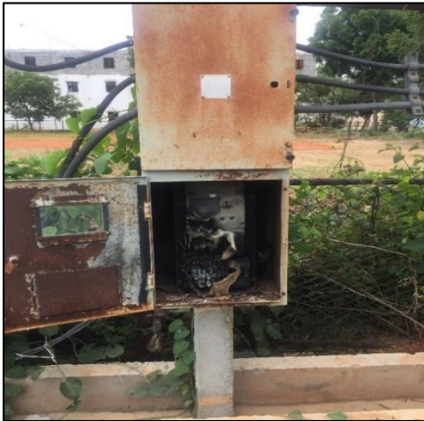
Figure 7: DT Meter burnt out (MBO)
