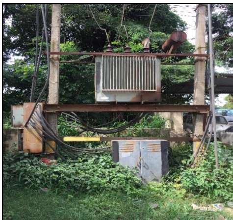
Figure 18: DT control box placed on ground
