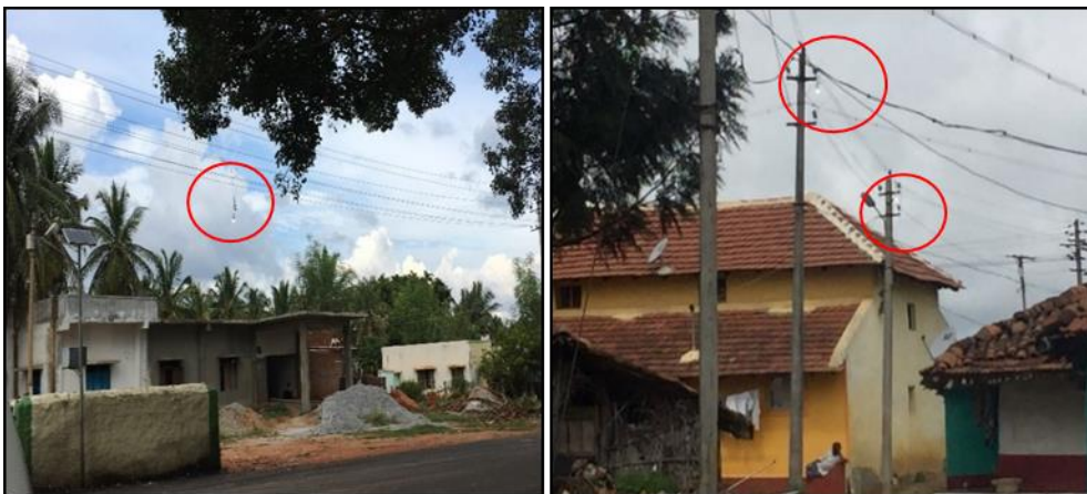
Figure 20: Unmetered street lights
