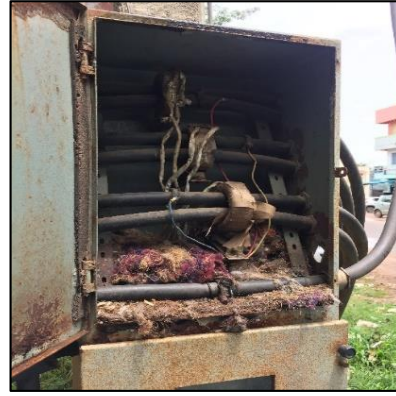
Figure 15: Burnt out connection in CT box
