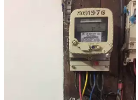
A tampered power meter
