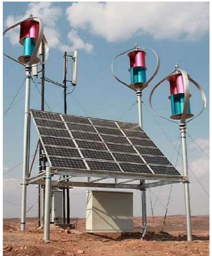
Solar Power System For Telecommunications
