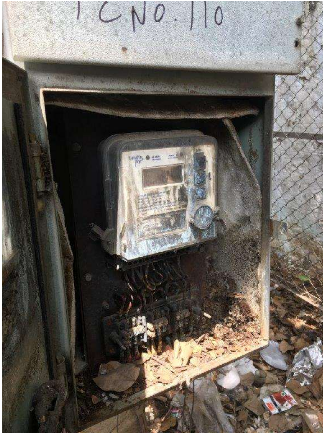
A burnt-out transformer meter. Pic Credit: Rishu Garg
